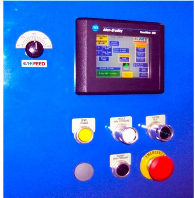
VERIFEED-Panel Mount shown top left next to other control panel components
